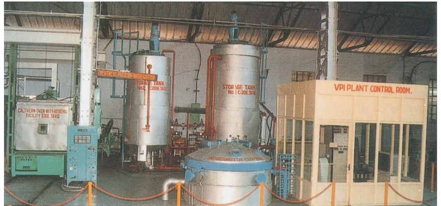
Vacuum Pressure & Impregnation Plant
